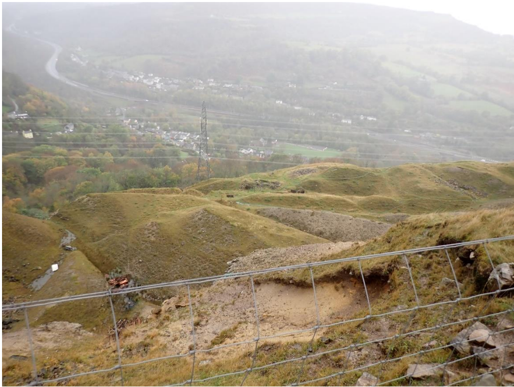
Plate 7: Chainage 69 to 79, The rock face / crest of slope moves within 0.5m of the back of the highway with surface slips on slope.
