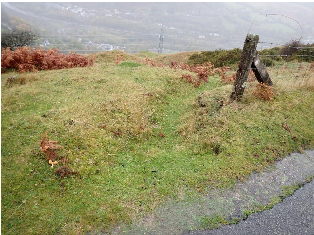
Plate 2: Chainage 6m. Grip in verge
