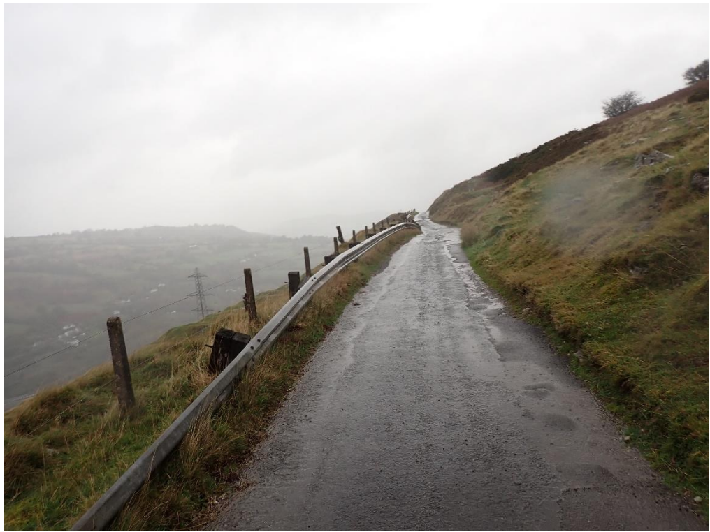
Plate 15: Chainage 104 to 112m, failed tilting VRS.
