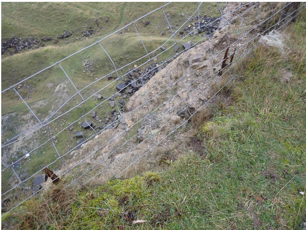
Plate 24: Chainage 215.0m, Section of fence with no support due to crest failure
