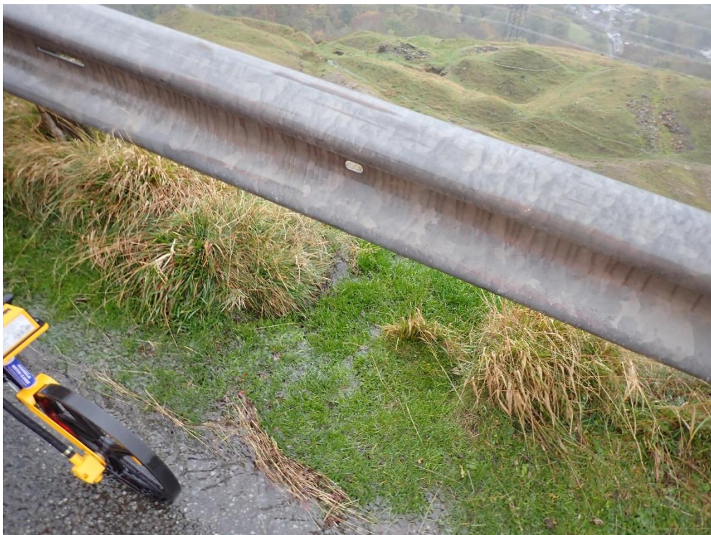
Plate 18: Chainage 139m, Low point in road, water draining off the road onto the failed slope below via a grip.
