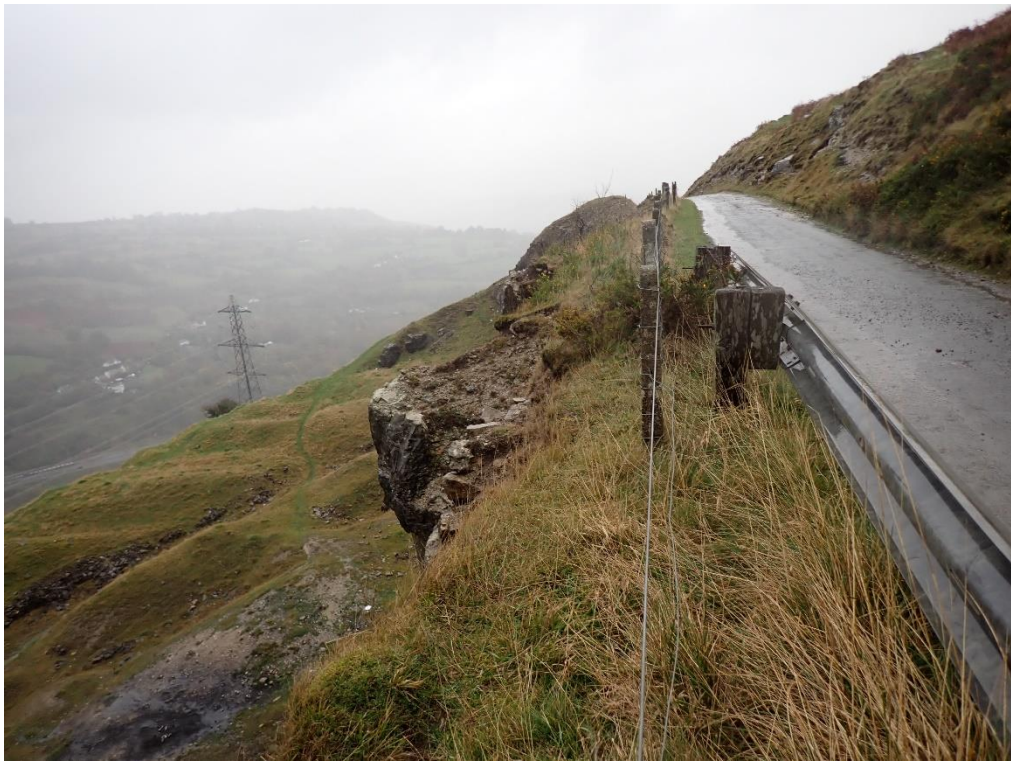
Plate 21: Chainage 179m, crest of slope / rock face close to edge of road. Note the end of the VRS at CH183.
