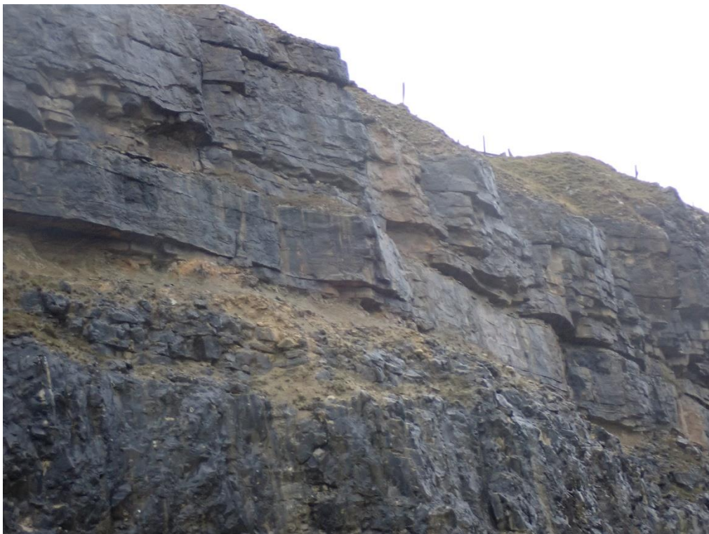
Plate 29: Weathering / erosion of the weaker material undercutting the upper section of the face.
