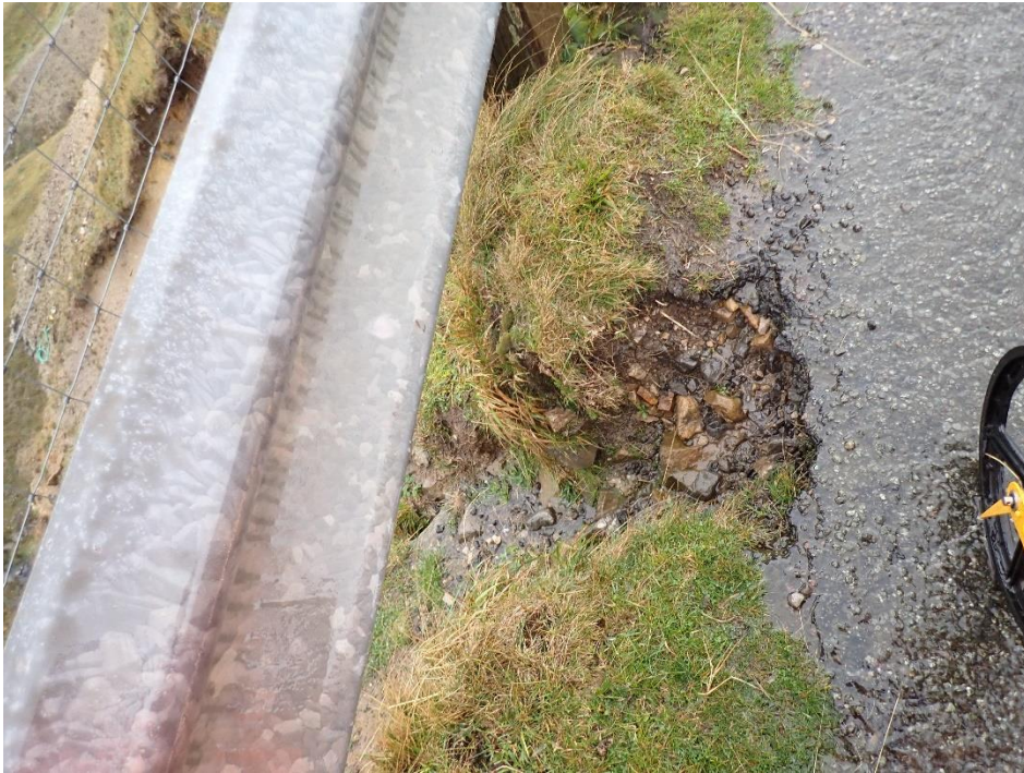
Plate 9: Chainage 74.5m Grip in verge.
