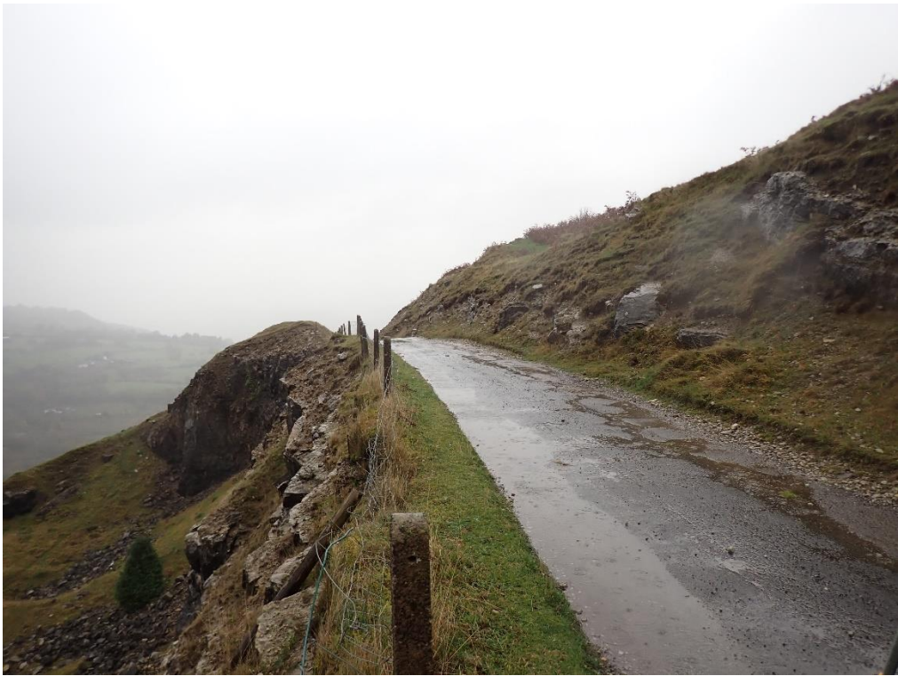
Plate 23: Chainage 202.0m, Failed section of fence
