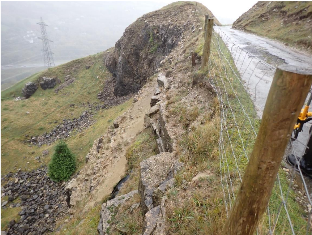
Plate 25: Chainage 228.0m to 250, Section of fence with no support due to crest failure
